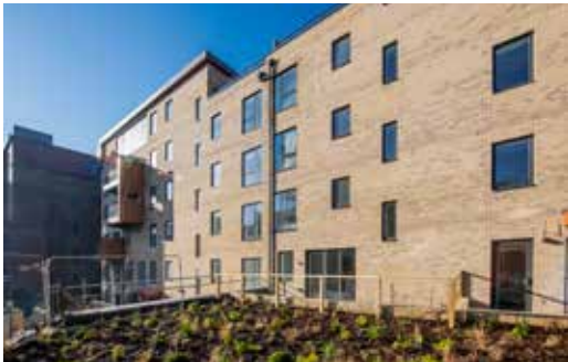
Photos of Tollgate Gardens taken in January 2020 as the works move towards completion.
