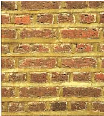
Careless pointing with strong cement mortar has caused irreversible damage to this eighteenth century brick façade (38 Upper Brook Street).
